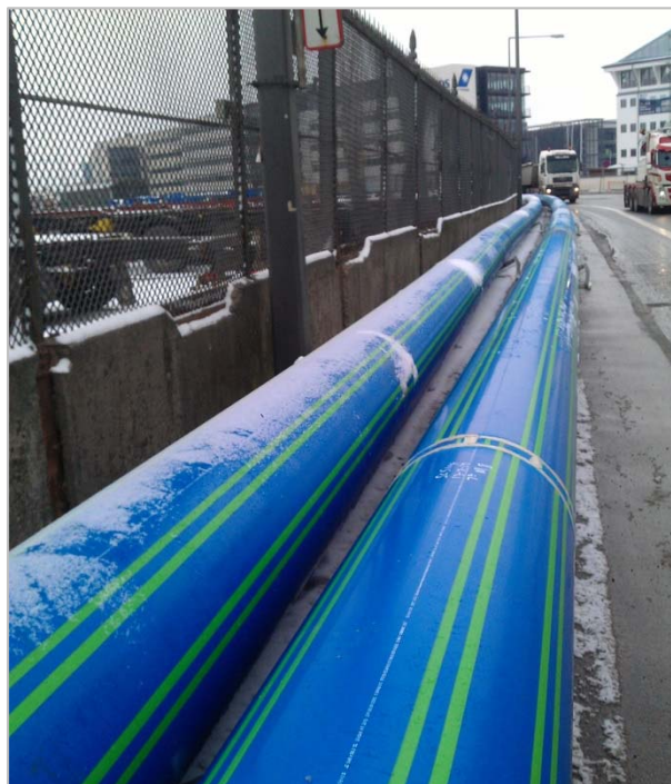
The pipe ends were butt welded together; the recoating of the weld area took place using the extrusion welding method.
